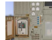
Power Conversion, & Distribution
